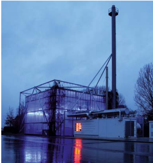
Co-generator powered by renewable raw materials
